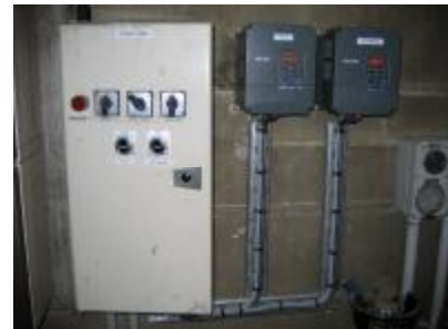
Two new variable speed drives were fitted (right)
