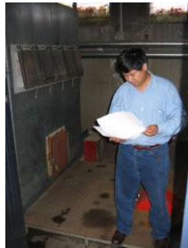
An audit of the boiler system identified the key issues of fuel and air supply rates and fire safety
