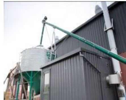
Radford Yarns wood pellet boiler house, fuel storage delivery system.
